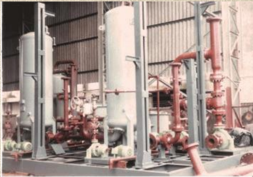
SKID MOUNTED CONDENSATE POLISHER PLATE WITH PIPING AND INSTRUMENTATION AND PUMPS ETC
